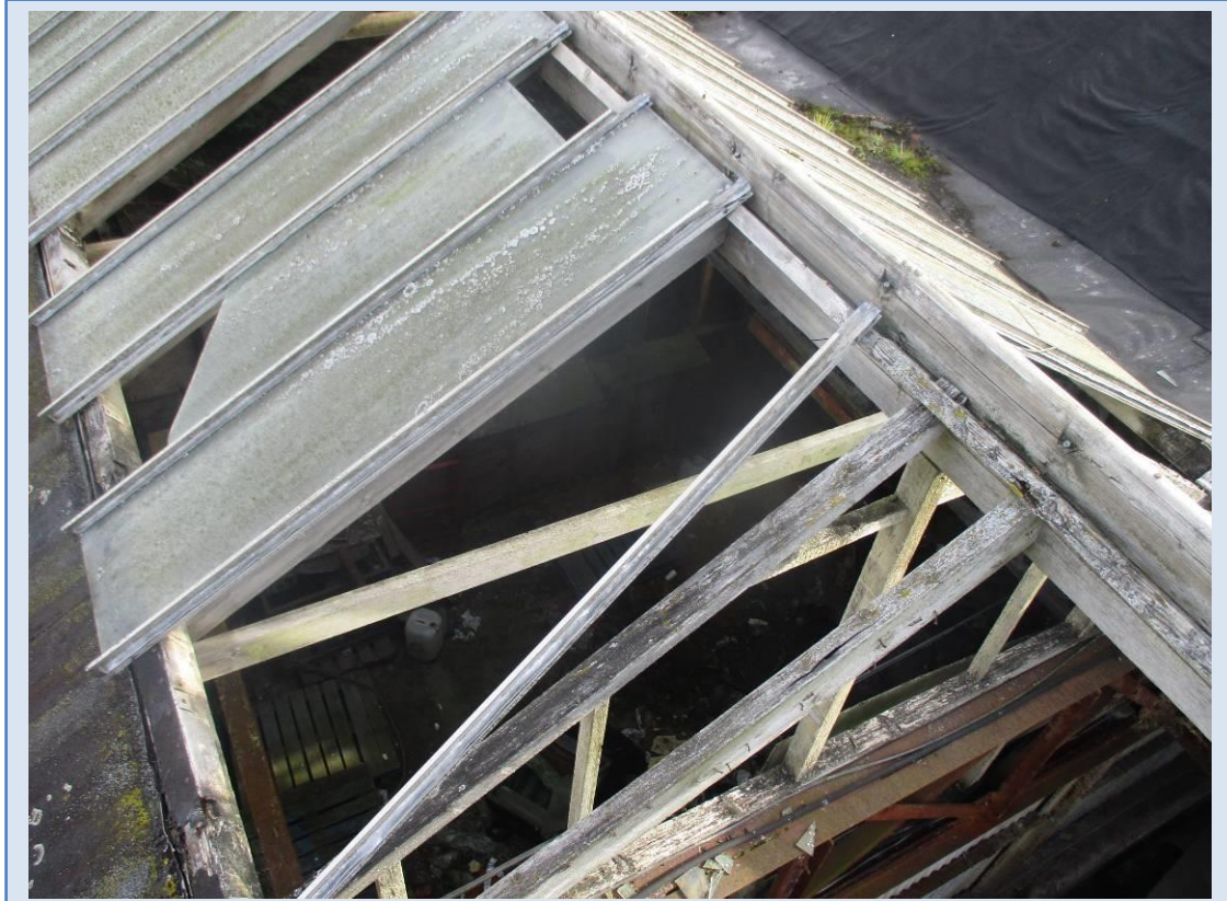
Asbestos containing rope seals debris internally in Building 1
