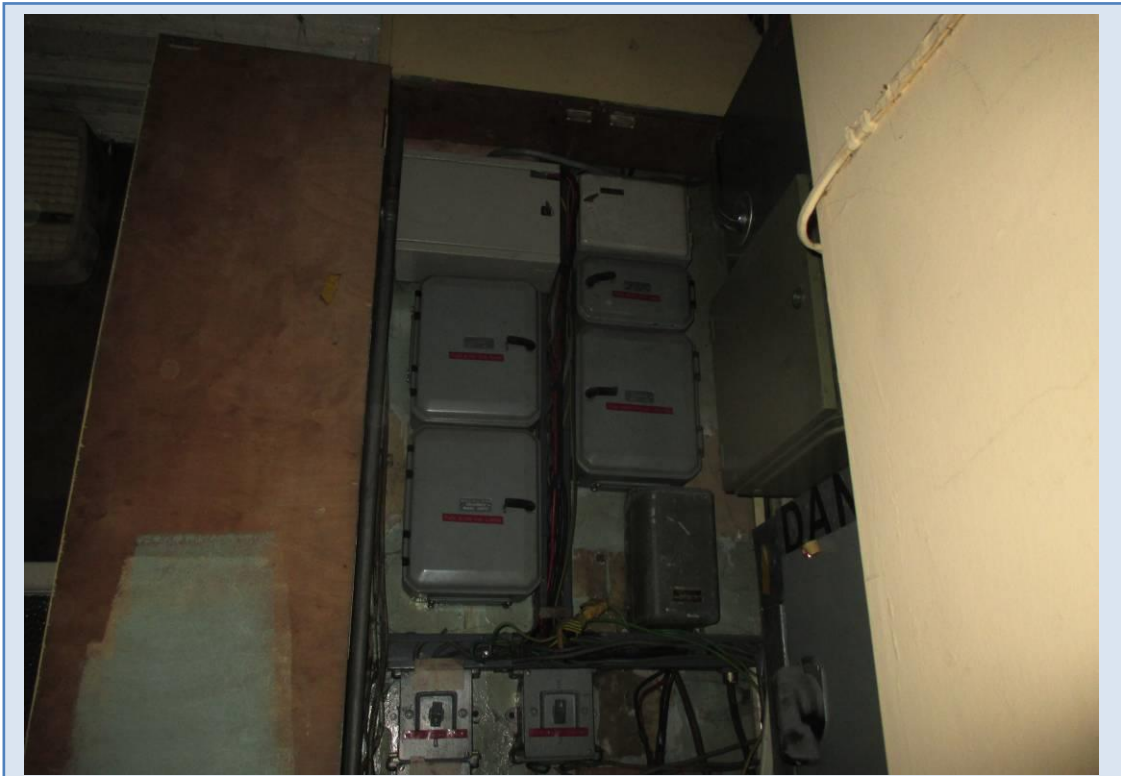
No inspection of live electrical or mechanical plant or similar requiring the attendance of a specialist engineer was carried out
