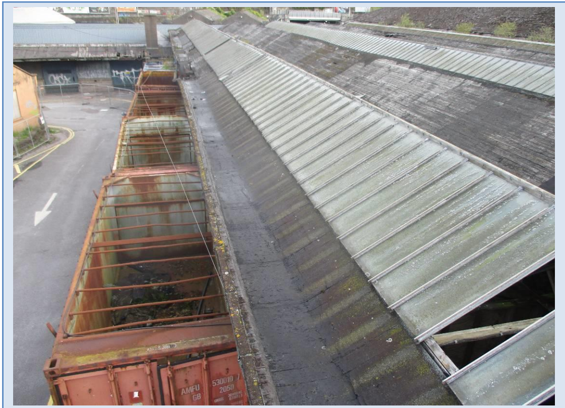
Asbestos containing rope seals behind the glazing bars of the roof lights on Building 1
