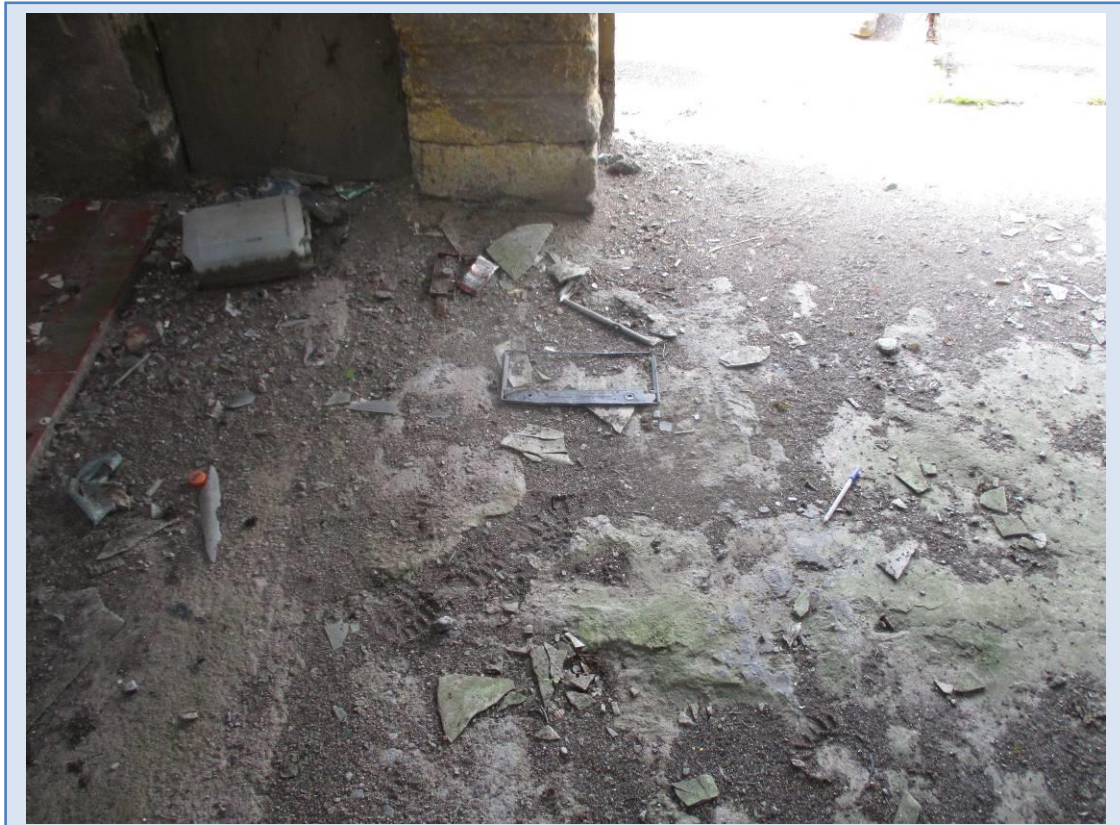
Asbestos cement sheeting debris in Building 7
